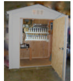
Ozone Groundwater Treatment- 45 gram/hr. 20 well injection system
